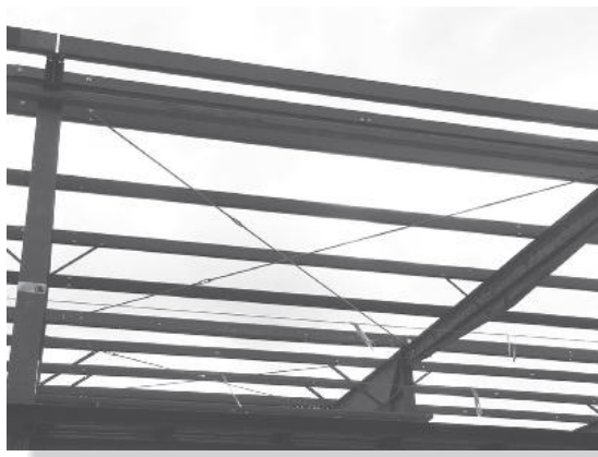
Tie rods are used for cross bracing to stiffen the roof of a building to resist wind loads.
