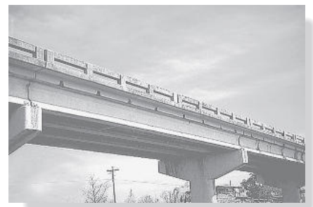
The prestressed concrete girders are simply supported on the piers and are used for this highway bridge.
